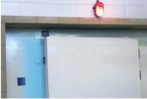
▲ Energy management of chilling rooms.
